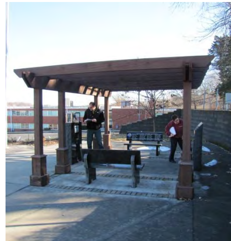
Image 4: The pergola over the monument is in need of additional maintenance.
