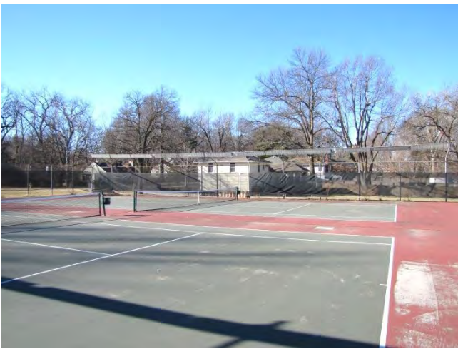
Image 1: The two tennis courts on site are in need of extensive repairs.
