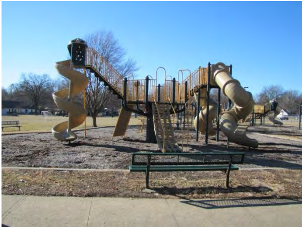
Image 1: Playgrounds and surfacing are in need of replacement to meet current ADA standards.
