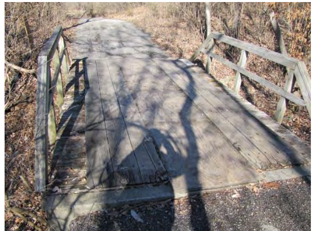
Image 2: The existing pedestrian bridge crossing has been temporarily patched; however significant safety concerns warrant full bridge replacement.
