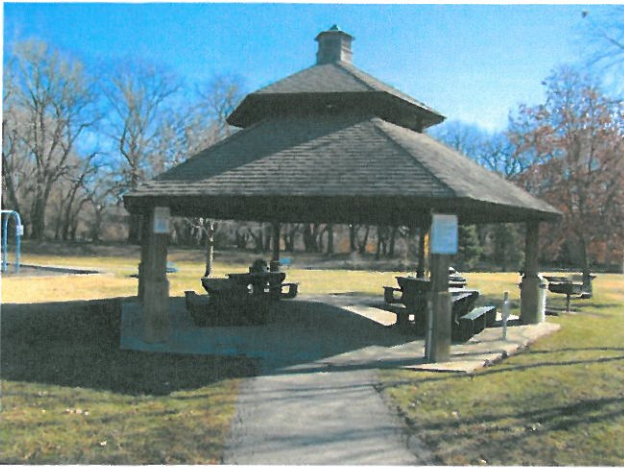
Image 5: The shelter structure on site is in need of maintenance. A larger shelter on site would support bigger community gatherings.
