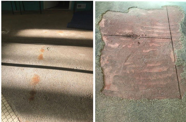
Oxidation through decking material; hydro-blasting overlay removal test area
