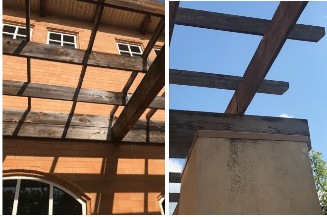
Discolored and weathered pergola; cracks & damage to cross members
