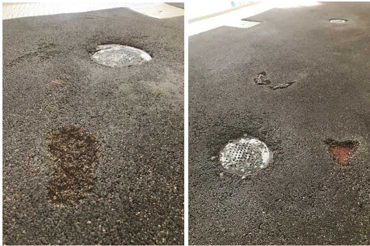
Deteriorating pool deck overlay material
