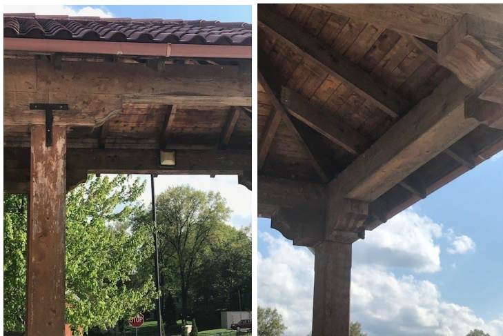
Southern breezeway damage; substantial woodwork preparation & staining
