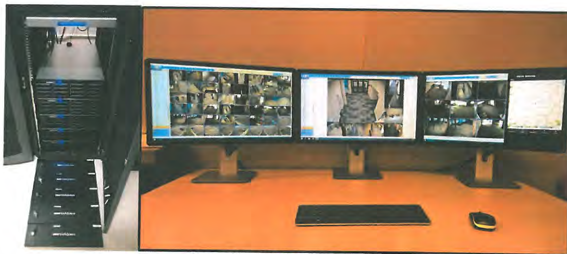
Server and Client Workstation installed by MDS
