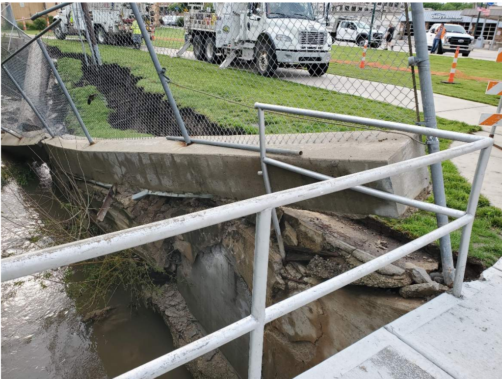
Figure A4: Looking west at eastern edge of failure.
