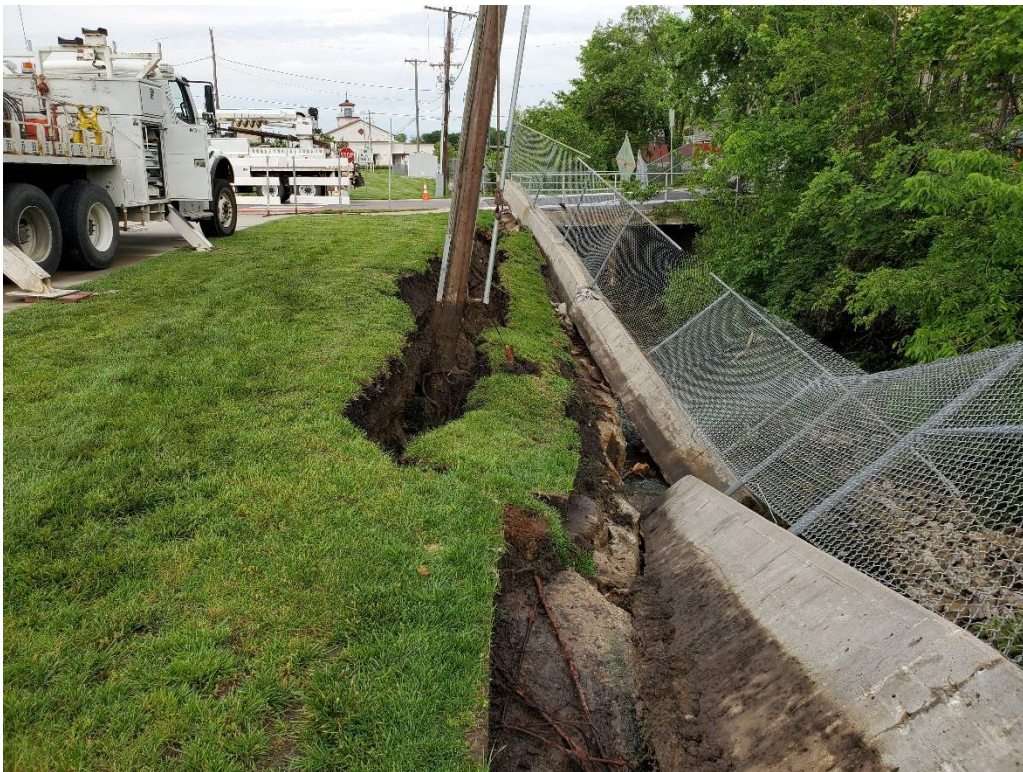
Figure A2: Looking east at failed retaining wall and Evergy pole.
