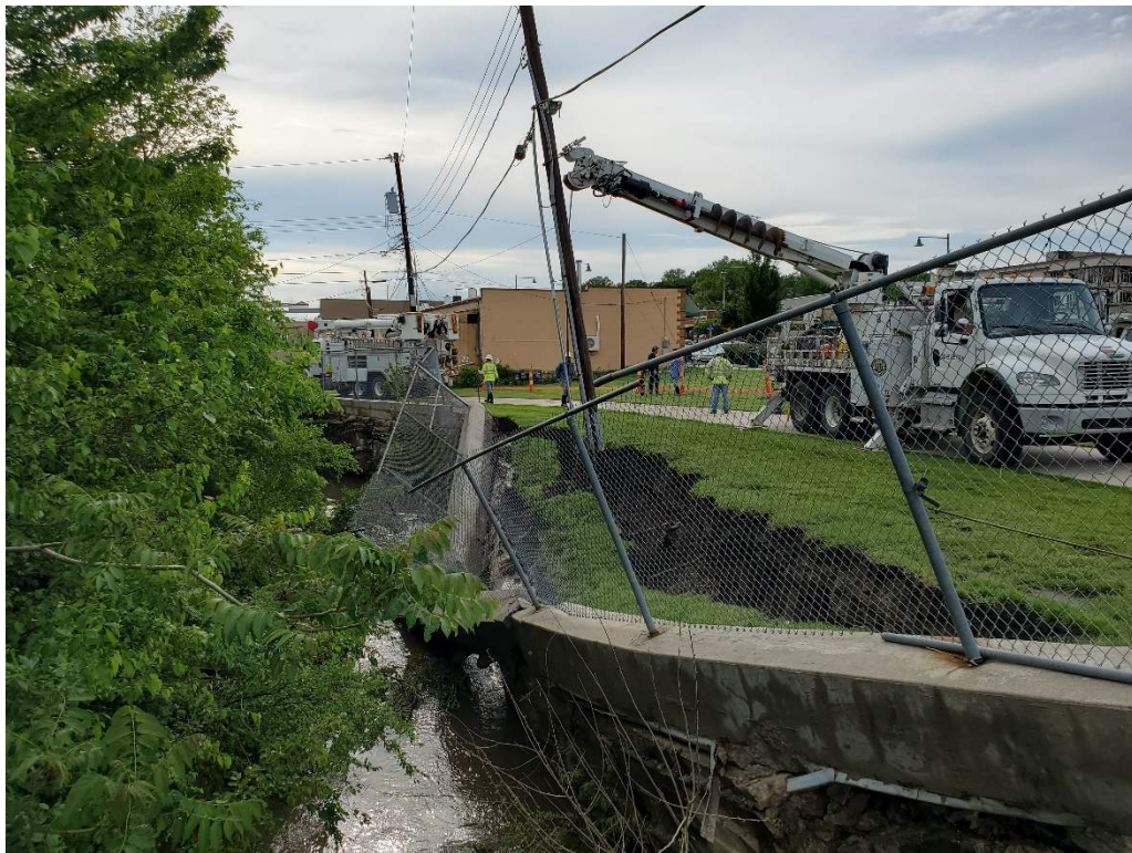
Figure 2: Looking west at failed retaining wall and creek (looking upstream of flow).
