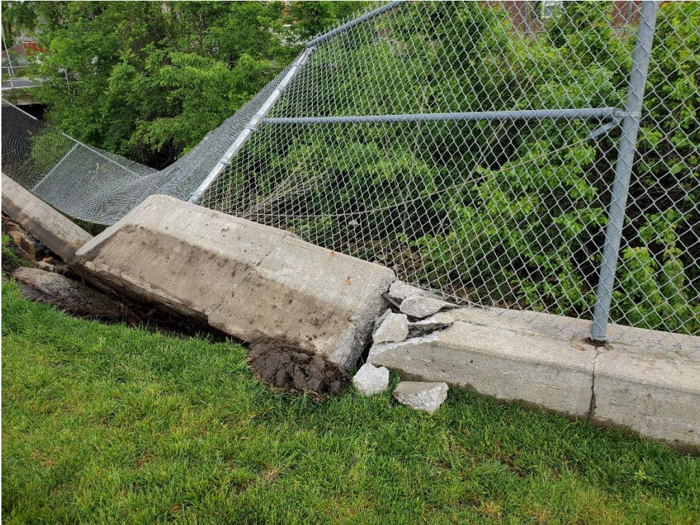
Figure A6: Closeup of western end of wall failure.
