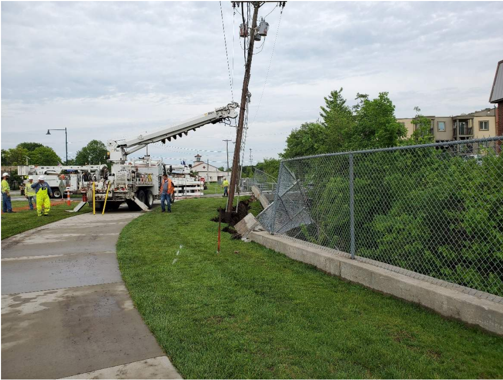
Figure A5: Looking east at failed wall with SS marked and new pole location staked.
