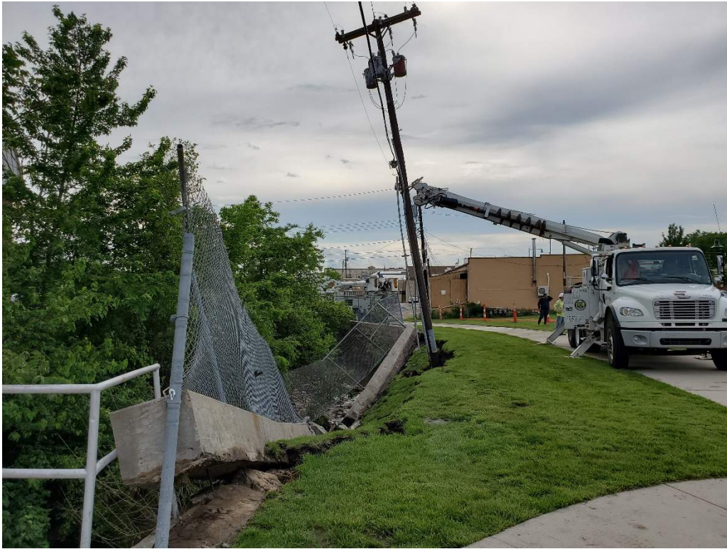
Figure A1: Looking west at failed retaining wall and Evergy pole that is being braced.
