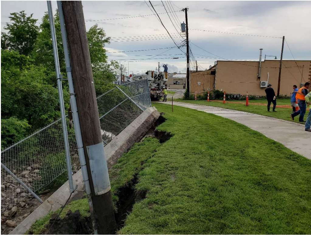
Figure A3: Looking west at western edge of failure.
