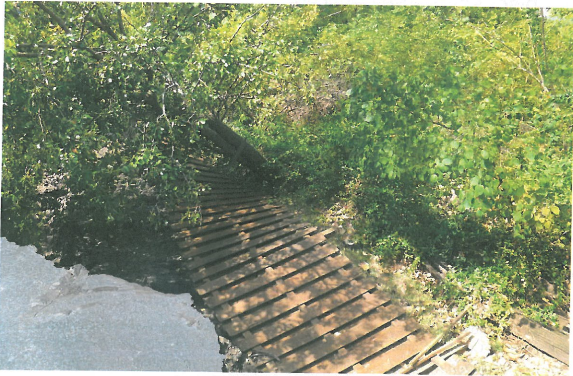
Figure 3. Photograph of Subsidence
