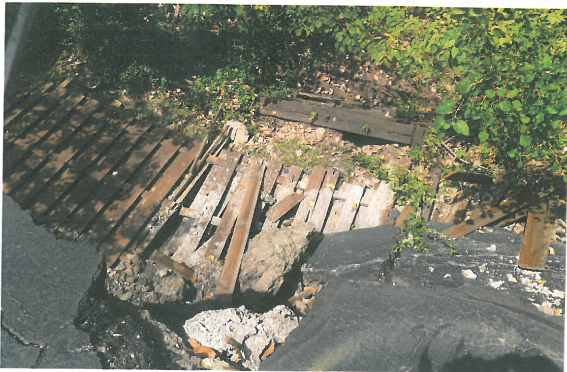
Figure 4. Photograph of Subsidence
