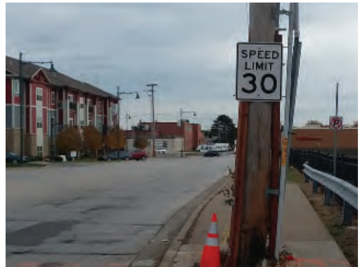
ISSUE: Sidewalk Obstacles on 61st Street adjacent to Target. Poles and other obstructions routine placed in sidewalks create additional obstacles, especially to users with disabilities.
